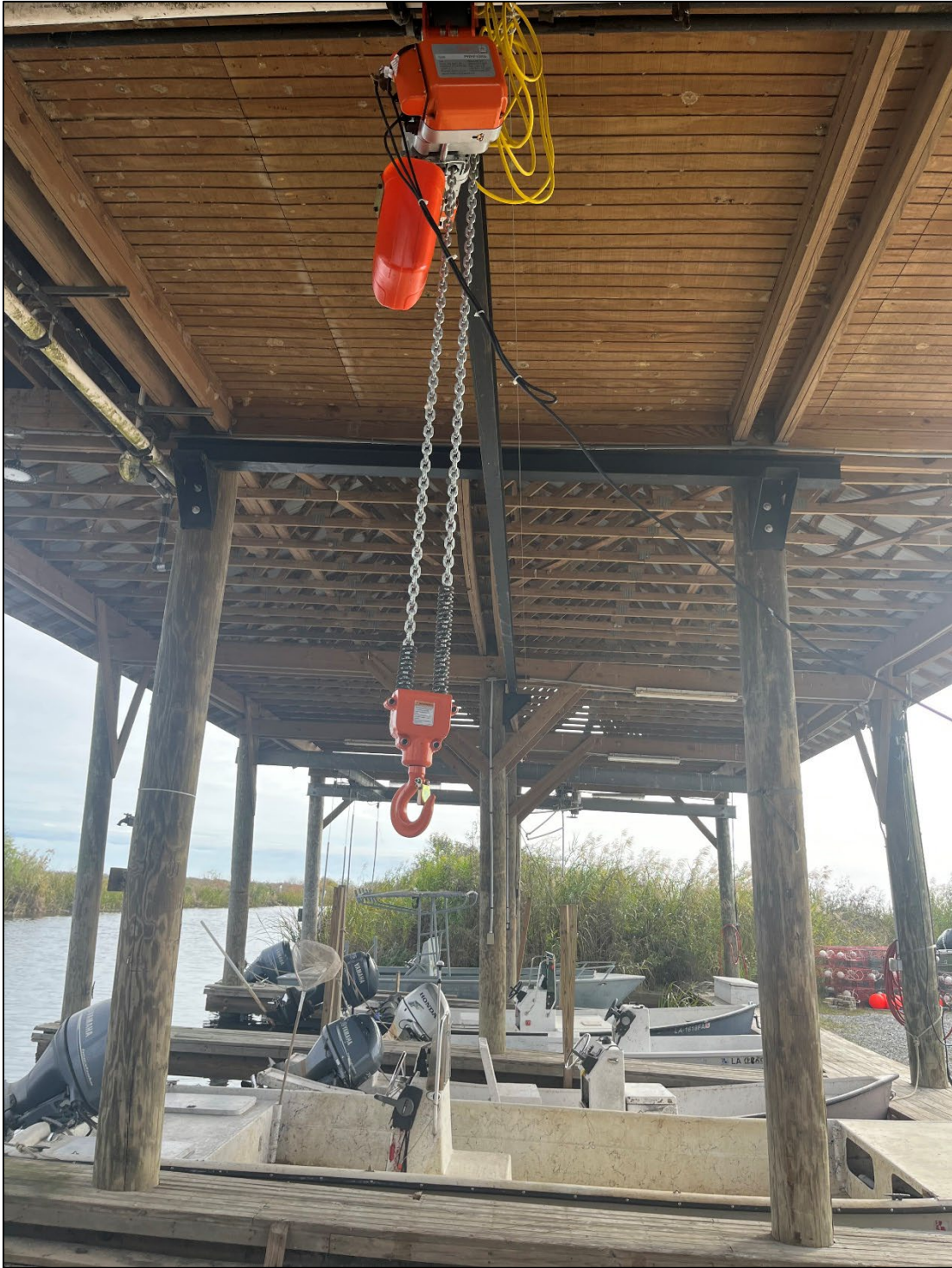
Appendix Figure 2. Newly installed winch/hoist system for buoy deployment at the Galva Canal Boatshed/Classroom Complex.
